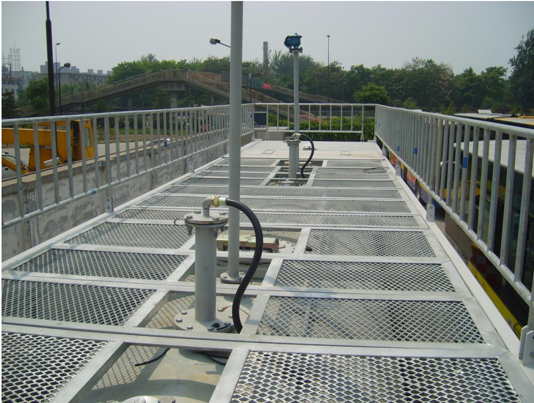
Above Ground Tank
